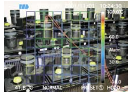
■ Maintenance of UPS and Batteries
