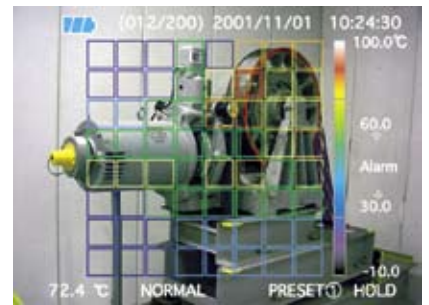
■ Maintenance of Moving Equipment, Such as Elevators
